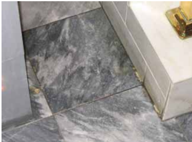
Here's the floor from page 78 before the repairs, and the scuff marks show someone hasn't learned that spike heels and a marble floor aren't exactly a good mix at the office, at home or anywhere.
