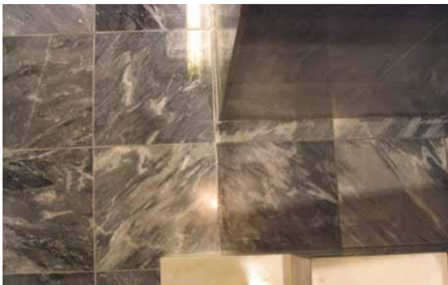
Take a look at the marble tiles on the right, and you'll see a fix that prevented a full tear-out of a law-office's floor; in low-light conditions, the honed floor with a color enhancer/sealer is barely noticed. But what warranted this kind of repair? (Photos courtesy TomMcNall)
